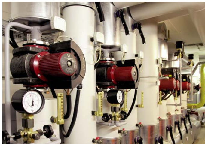
One of the low-investment energy-saving measures is checking the hydraulics and the pump runtimes.
