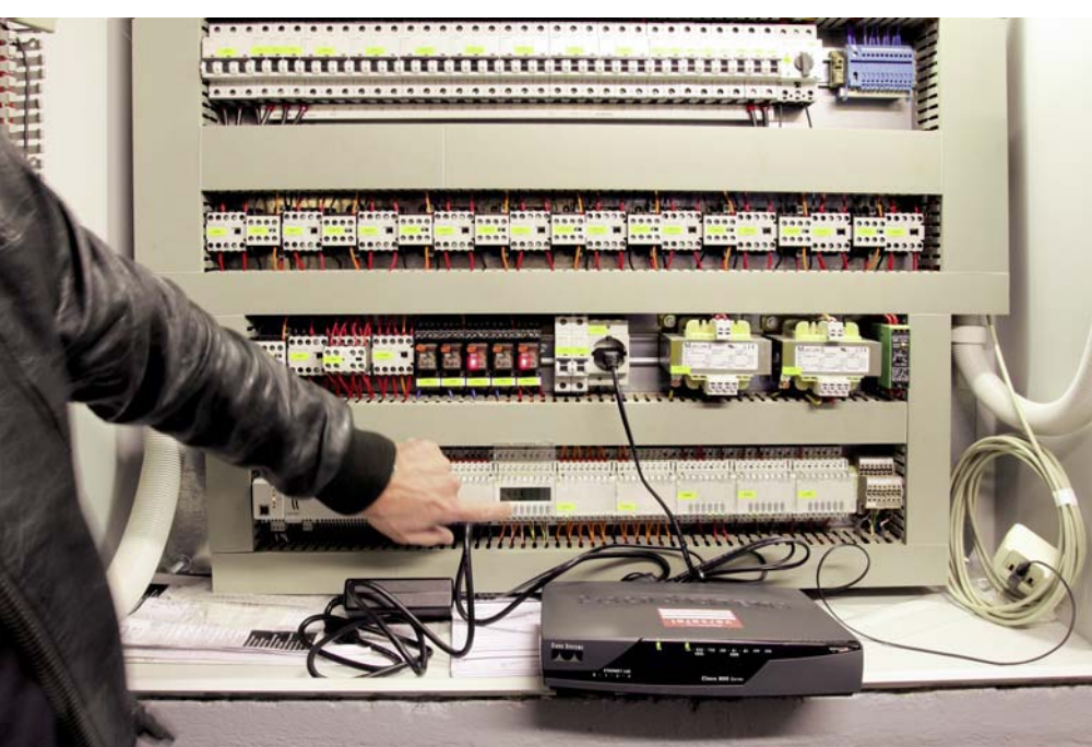
The interface between the on-site controlling and the control centre is taken over by a DSL router (Cisco) which is provided by the telecommunications provider Versatel.
