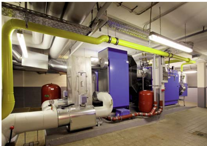
Wherever it is possible and economical, gas and heating meters with a meter pulse are re-fitted to monitor the efficiency of the boilers.
